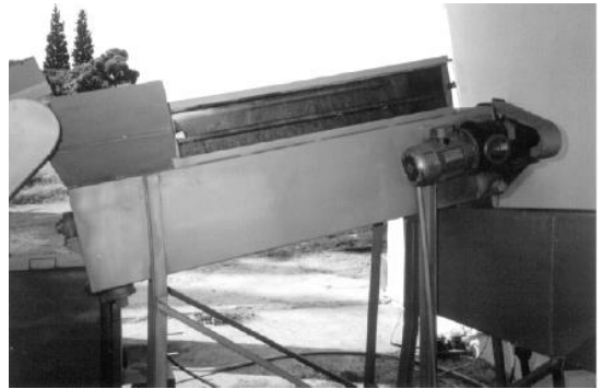
Picture 4. Acid spraying system.
